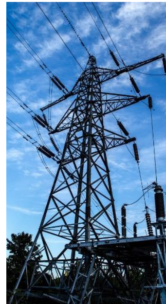
Hoogspanningsmast. Bron: Windpowerengineering.com
